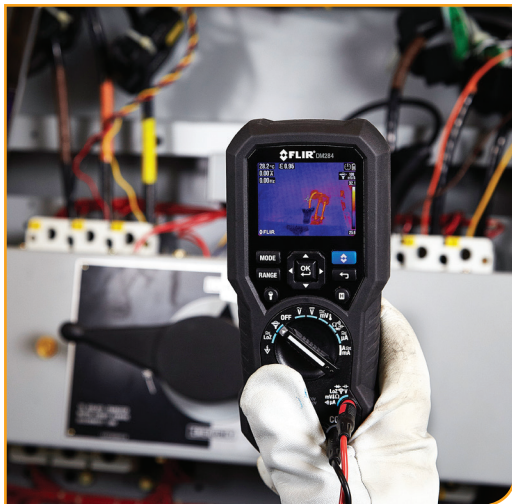
Thermal scan of an electrical panel
