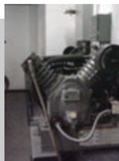
Air Compressor – Full Visible
