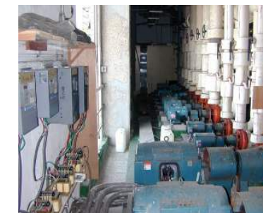
Air Conditioning System
